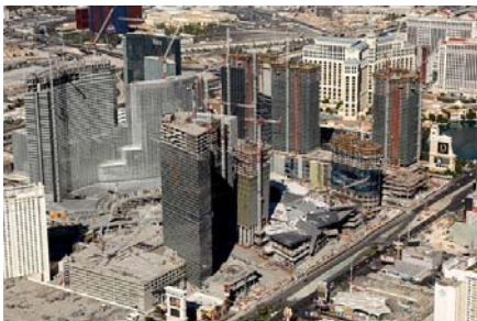
An aerial view of the construction site for CityCenter on Nov. 6 in Las Vegas.
